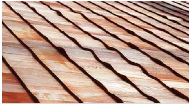
Figure 5. Buckling of shingles installed with insufficient space between adjacent shakes/shingles to accommodate swelling.
